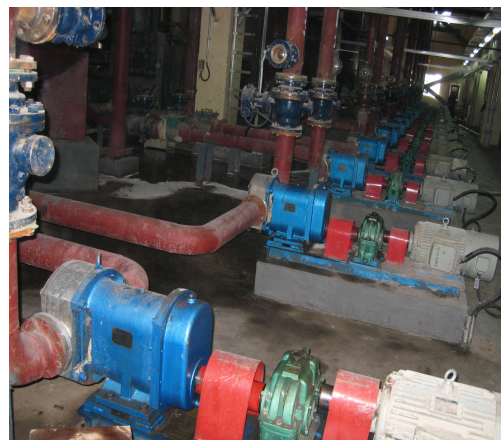
Chemical fiber factory slurry transport pump
