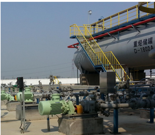
Rotor pump delivery heavy hydrocarbon
