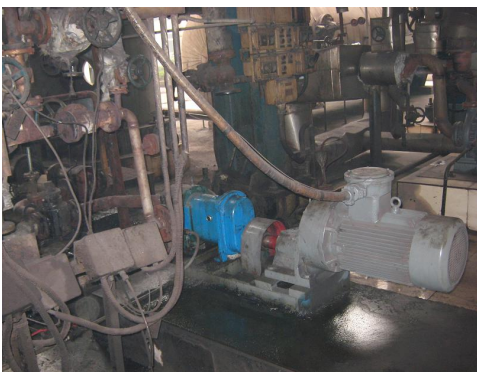
Rotor pump conveying high temperature coal tar in coking plant coal (≤320°C)
