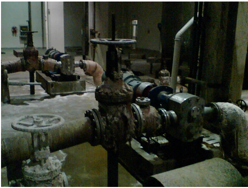
Chemical fiber factory slurry transport pump
